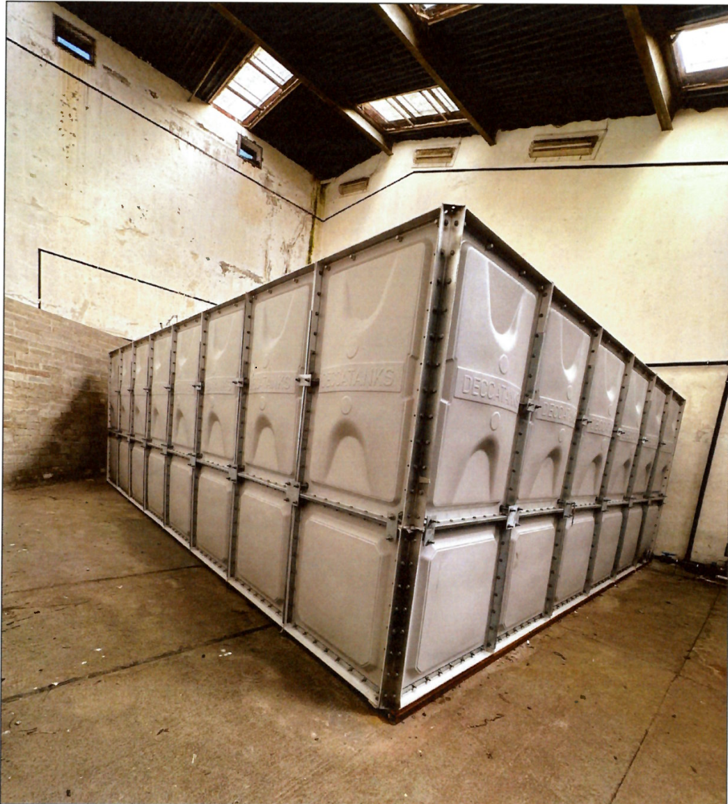
Figure 2.4: Subject water tank located within disused handball courts building. (Source: IMAC Group, 2025).
