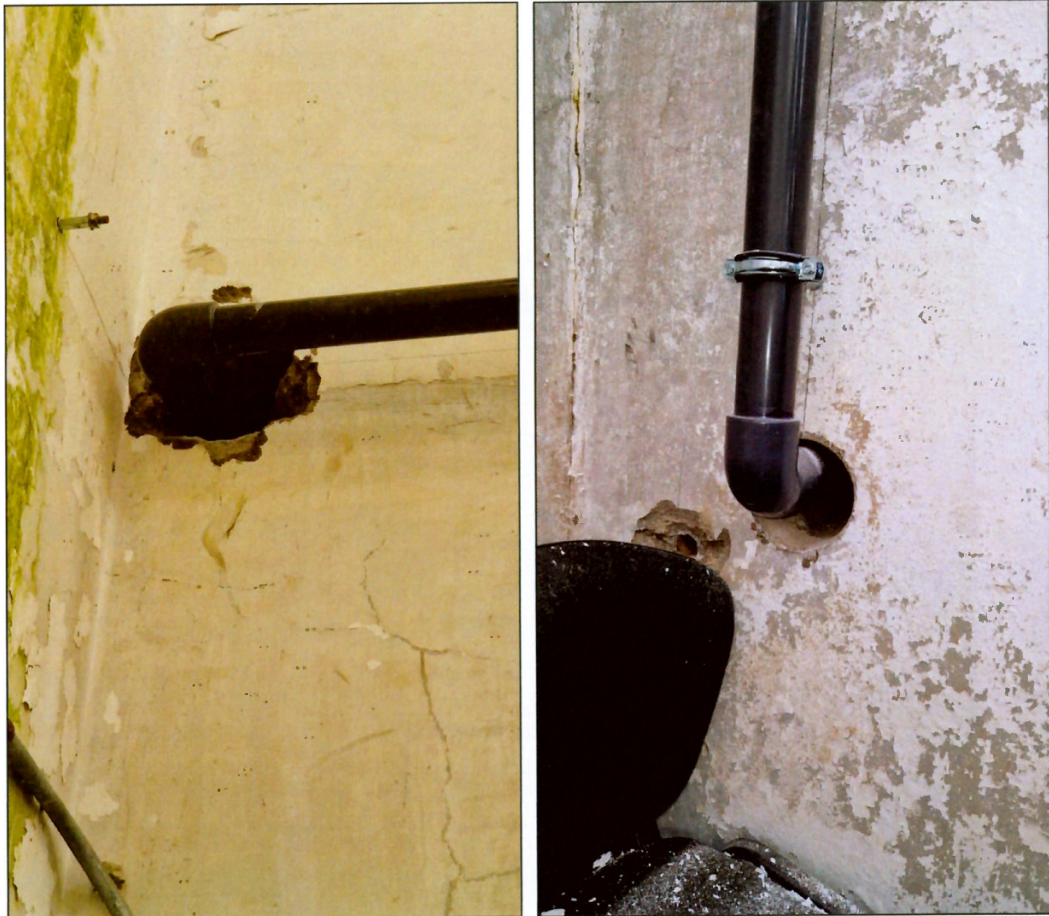
Figure 2.5 and Figure 2.6: Bored holes in walls of disused handball courts. (Source: IMAC Group, 2025).
