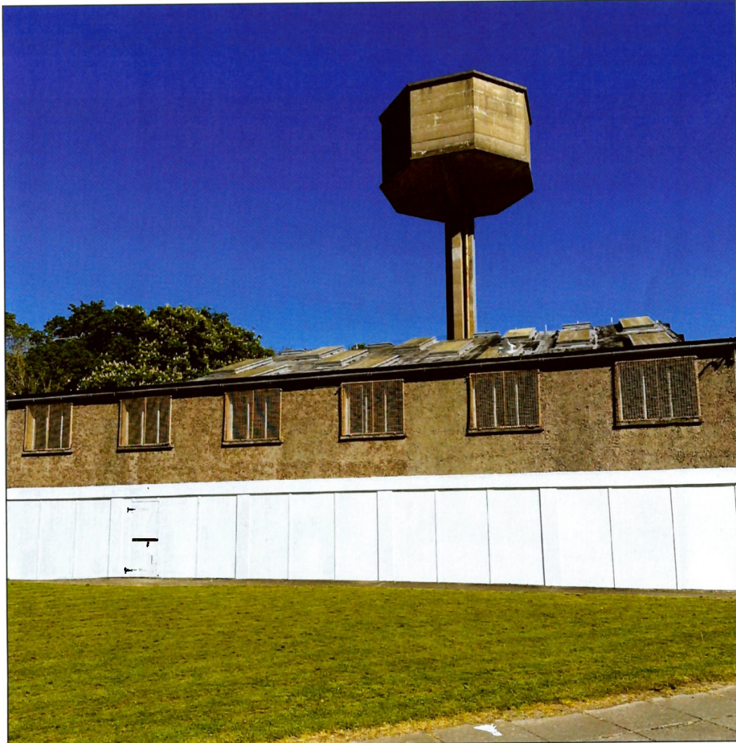
Figure 2.3: Exterior of disused indoor handball courts in which the subject water tank is located. (Source: IMAC Group, 2025).
